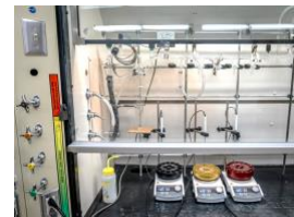
Fume hood sash shielding
